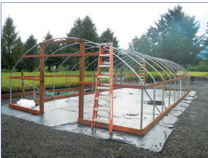
Figure 13. Shade house being constructed at the Oregon Youth Authority Camp Tillamook Work Study Center to use for direct sowing and outdoor natural stratification over the winter. The shade cloth protects seed from bird and rodent predation yet allows for ambient temperatures and rain. (Photo by Kurt Heckerroth 2012)
